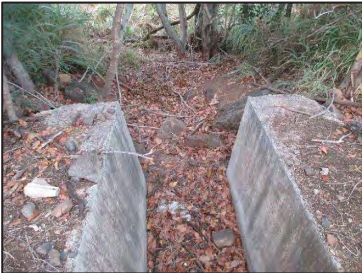
Photograph 1. A view of tank discharge point/headwall to the drainage ditch. The DU was 12 ft wide by 100 ft long. The width of the drainage ditch varied (27 June 2018).
