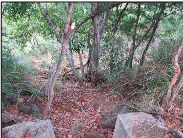
Photograph 2. A view of DU1 just beyond the discharge point. The drainage ditch was covered with vegetation, boulders, and rock. The DU was 12 ft wide by 100 ft long. The width of the drainage ditch varied (27 June 2018).
