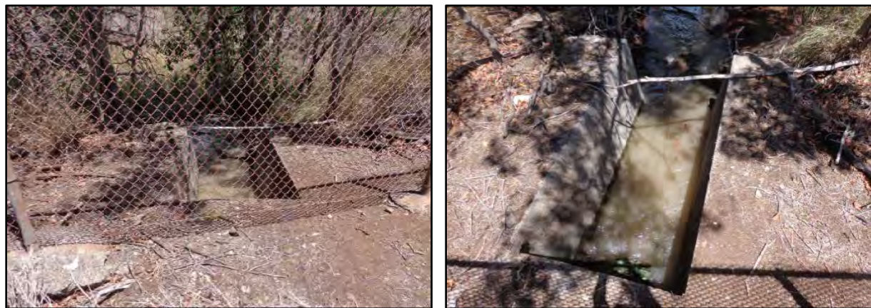
Photographs taken during tank flushing, following an inspection of the tank interior (August 2017)
