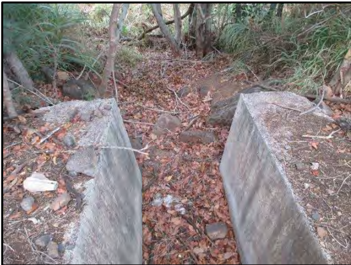
Photograph 1. A view of tank discharge point/headwall to the drainage ditch. The DU was 12 ft wide by 100 ft long. The width of the drainage ditch varied (27 June 2018).
