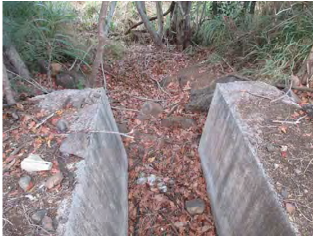
Photo 1: Reservoir discharge outlet
