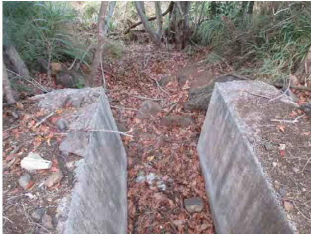
Photo 1: Reservoir discharge outlet
